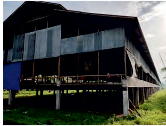
Figure 9.6. High Rised Poultry House.
